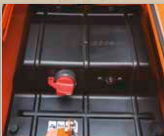
Battery cut-off switch
